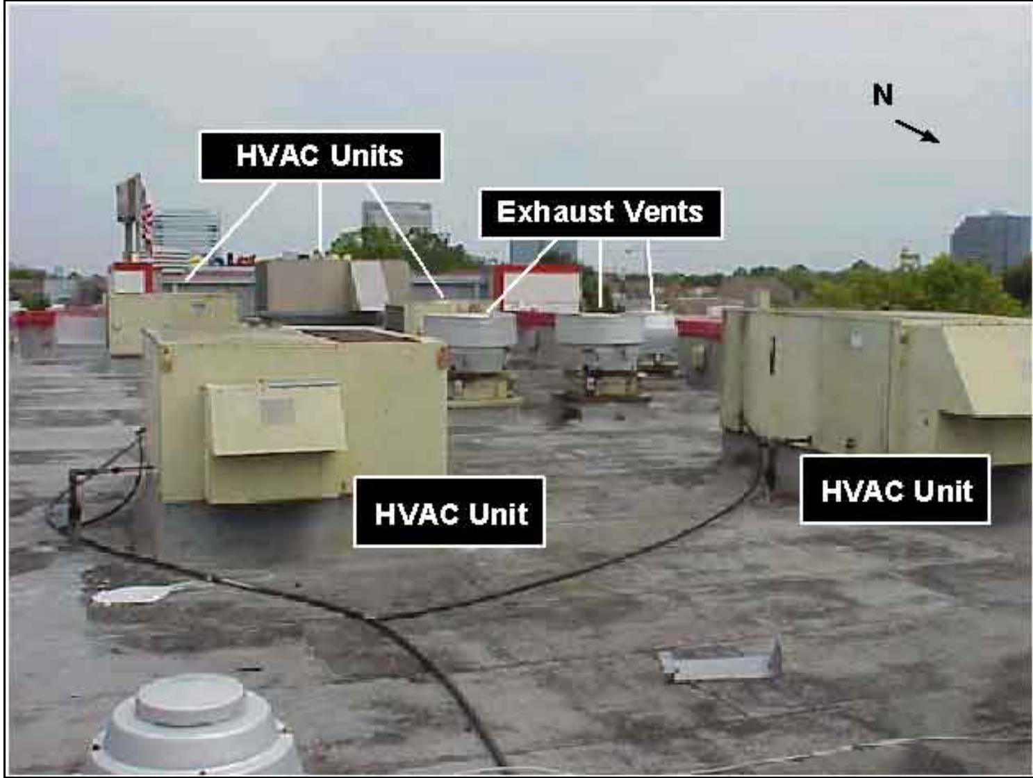
Photo 2. HVAC Units and Cooking Vents Positioned on the Roof of the Restaurant Note: Photo was taken of a restaurant similar to the one involved in this incident.
